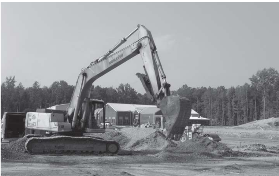
Construction is underway on the Trades School on Learning Lane. The Trades School will be ready for students next fall.
